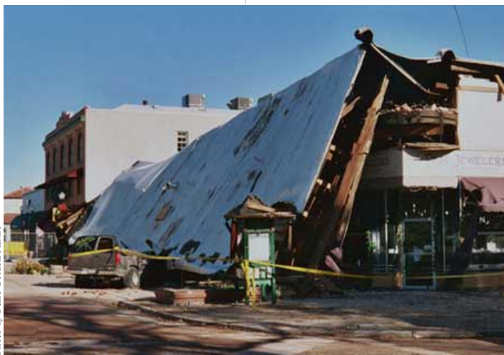
Historic structures and a vehicle were damaged in Paso Robles from January's 6.5 San Simeon quake.
